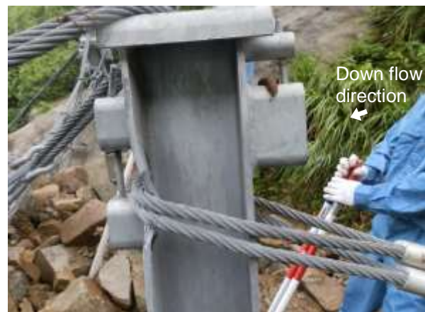
Fig. 20 Deformation of the post head
