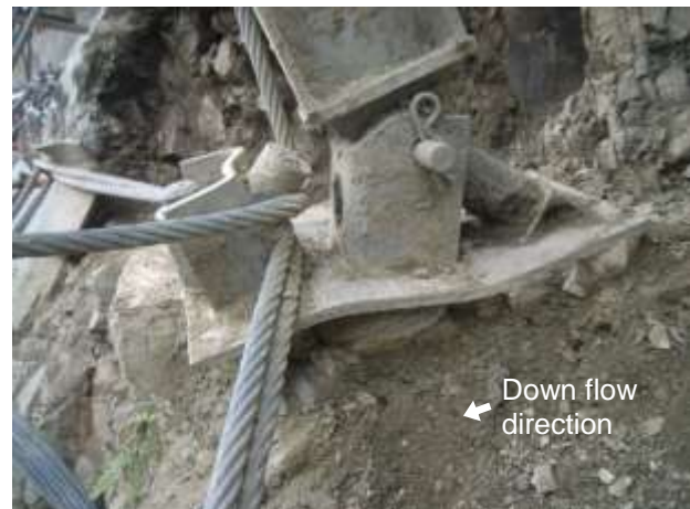
Fig. 21 Deformation of the base plate
