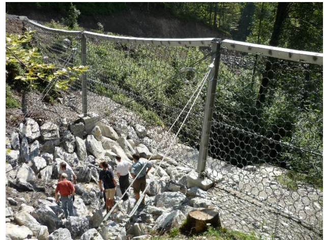
Figure 2: UX debris flow barrier, with posts for wider stream channels application. Example of the Trachtbach in Switzerland. Additional scour protection, rip-rap and lean concrete were placed along the stream bed.
