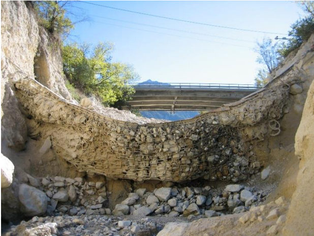
Figure 1: Testing of debris flow retention system with ring net in the Illgraben channel, 2006. Retention volume approx. 1000 m 3
