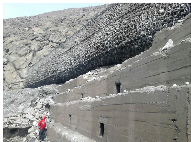
Figure 11: Filled debris flow barrier in 2017 in Peru, protecting successfully a large city downstream.
