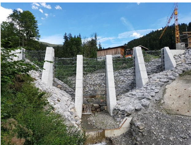
Figure 13: Another special construction acting as a debris flow
