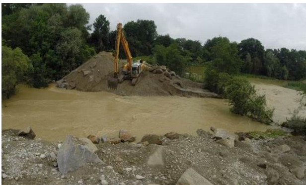
Fig. 2 Artificial levee breach (Source: VERBUND Innkraftwerke GmbH)
