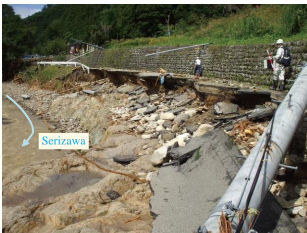
Fig. 7 Municipal road washed
