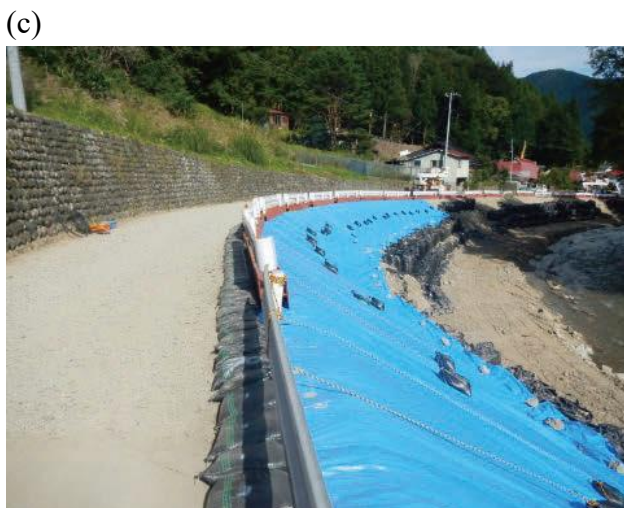
Fig. 14 Removing obstacles from the road (a) Removing sediment and driftwood (b) Damaged areas are temporarily repaired with large sandbags (c) Road temporarily restored
