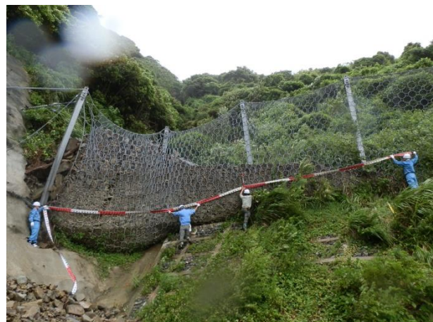
Photo 4 An example of capture of debris by the flexible debris flow barriers
