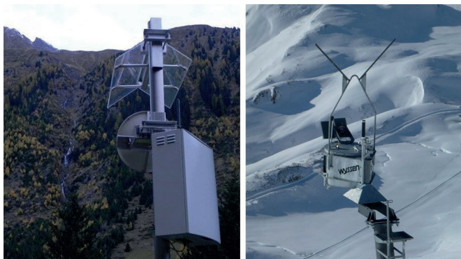
Figure 2: A LARA (left) and a SARA (right) installation used for avalanche detection for operational road protection.
