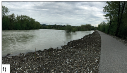
Figure 1f: Flood mitigation and restoration project Aare River: left bank widening flood discharge
