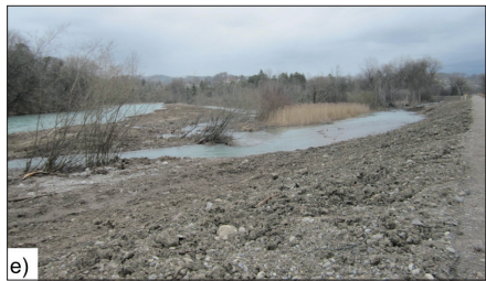
Figure 1e: Flood mitigation and restoration project Aare River: left bank widening normal discharge
