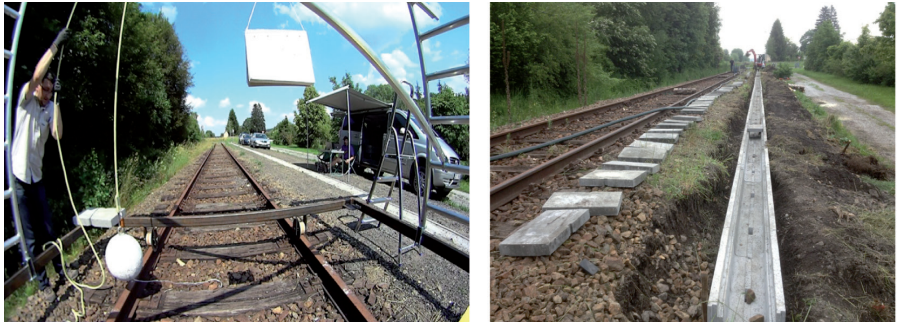
Figure 2: Left: impact on rails with a granite bowl from a predefined drop height. Right: Installation of cable trough according to OEBB regulations for the field experiments.
