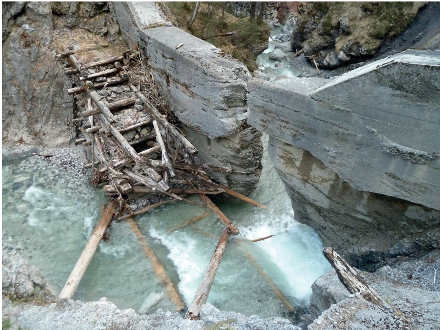
Figure 4: A degraded check dam on the Belca torrent in NW Slovenia.
