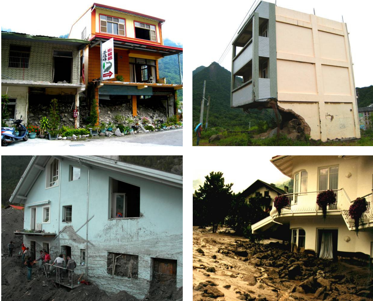
Fig. 4 Typical damage patterns for buildings affected by torrent processes in Taiwan (top) and Austria (bottom). Upper left: Songhe community, Taiwan, event of August 2004, upper right: Min-Zu community, Taiwan, event of August 2009, lower left: Pfunds community, Austria, event of August 2005, lower right: Wartschensiedlung village, event of August 1997. Credits: upper left: S. Fuchs (27 August 2011), upper right: S. Fuchs (28 August 2011), lower left: Gebietsbauleitung 6.2 (23 August 2005), lower right: anonymous (event of 16 August 1997).
