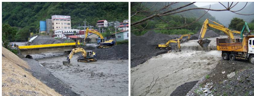
Fig. 10 Heavy machinery standby along Nantou DF012 torrent during Typhoon Morakot, 2009 (photo by Sinotech, INC.)
