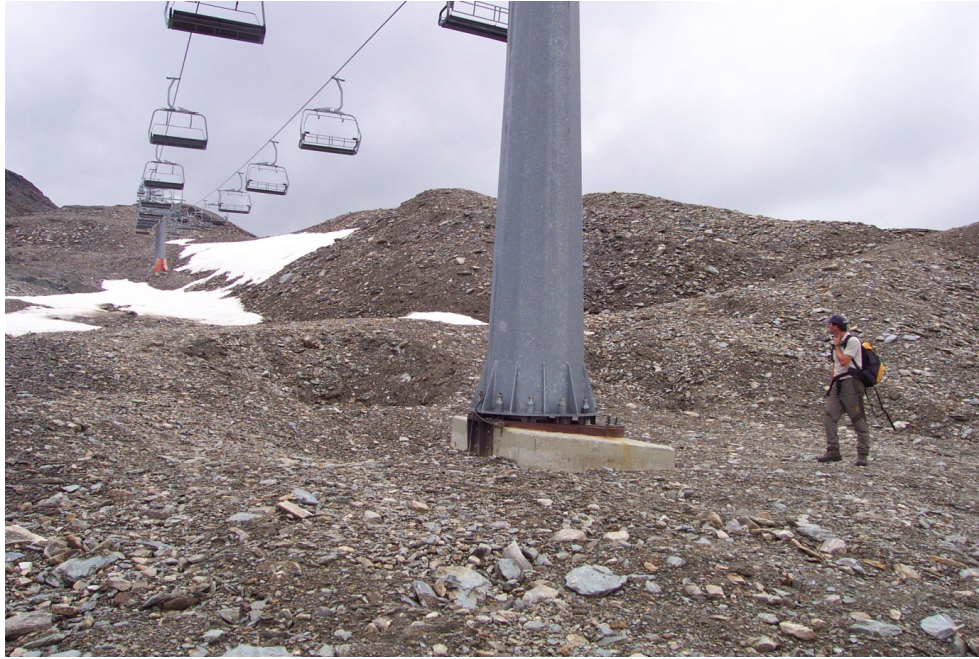
Fig. 3 Soil subsidence in the vicinity of pillar no. 12 of the ski lift "Madritschjoch" and re-adjustment of the position. Note the inclined foundation of the pillar.
