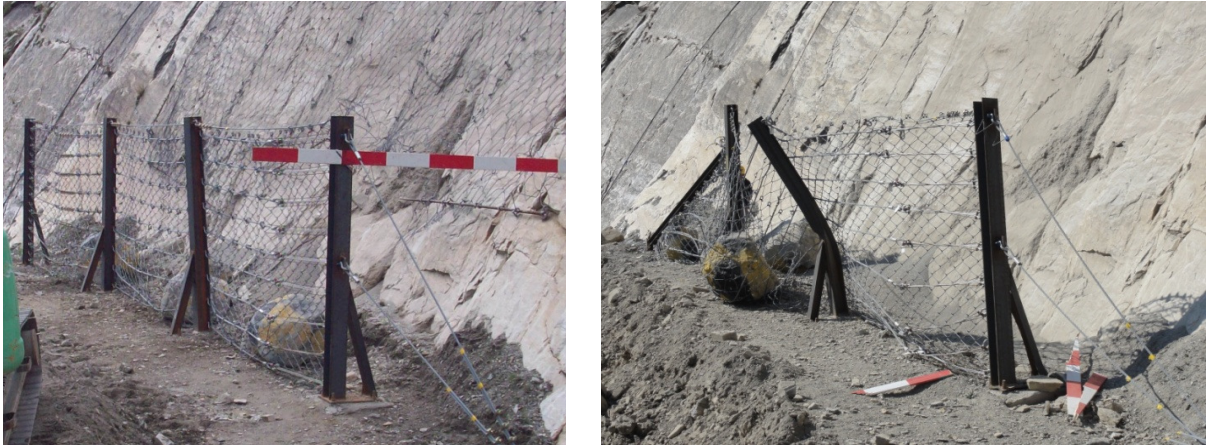
Figs. 9 (left) low deflection barrier with rock fall attenuator protection (20 attenuated impacts), (right) low deflection barrier after 8 un-attenuated impacts during the rock rolling experiments
