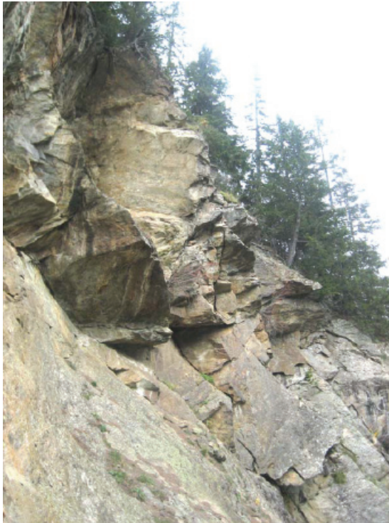
Fig. 6: Detachment area of Versahl, Area B with orthogneises showing loose rock conditions, low joint strength and unfavourable joint orientation. As the relevant detachment mechanism gliding is considered.
