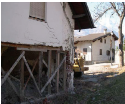
Fig. 4 : Oct. 2000 – Nus, house hit by the debris
