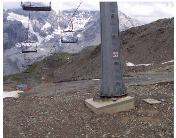
Soil subsidence and subsequent adjustments of foundation. Photo: A. Zischg
