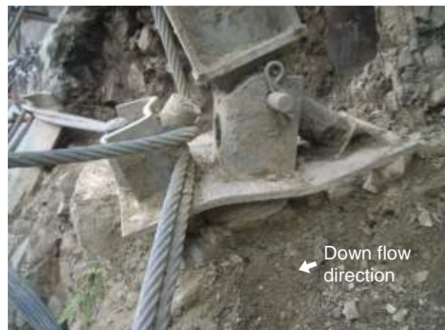
Fig. 21 Deformation of the base plate
