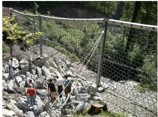
Figure 2: UX debris flow barrier, with posts for wider stream channels application. Example of the Trachtbach in Switzerland. Additional scour protection, rip-rap and lean concrete were placed along the stream bed.
