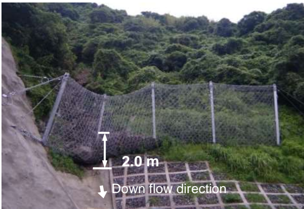
Fig. 7 Capture case of collapsed sediment (a)
