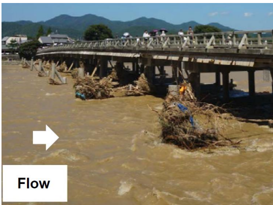
Fig. 2 Stakes at Togetsu Bridge during a 2013 flood [Takebayashi, 2014]
