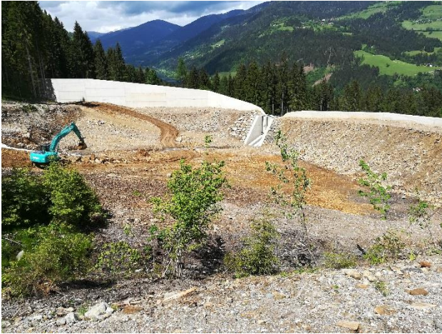
Fig. 11 Bedload sorting dam with a retention capacity of 37,000 m 3 with a length of 250 m and a height up to 14 m
