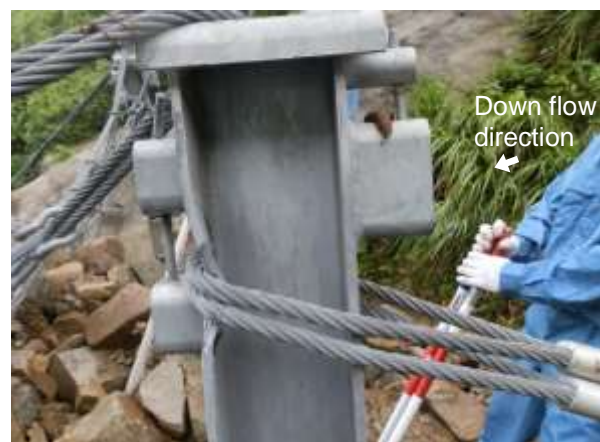
Fig. 20 Deformation of the post head
