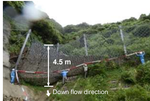
Fig. 8 Capture case of collapsed sediment (b)
