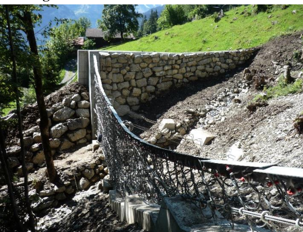
Figure 9: Debris flow barrier in Isenflue above a settlement. The outer bank of the stream was reinforced with a rock wall.
