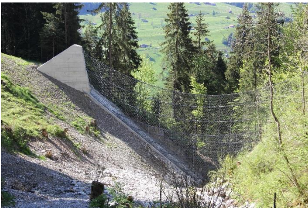
Figure 12: Special construction of a debris flow barrier in Hüpach, in Switzerland, with a width of 40m and a netting height of 10m.
