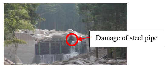
Fig. 2 Damage of steel open dam by large rocks
