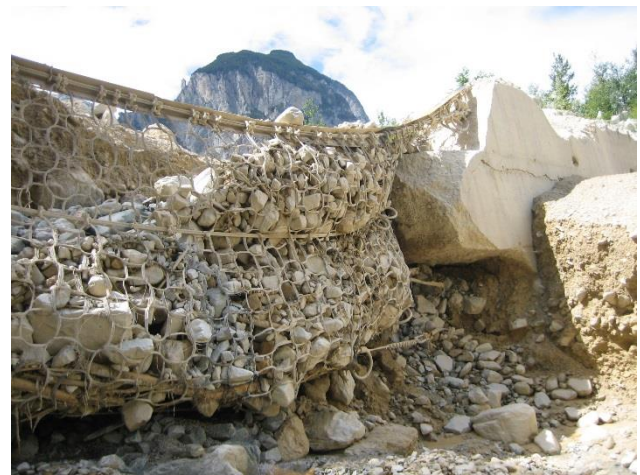
Figure 5: Washed out anchoring of the debris flow barrier number 25 in the Illgraben channel. Anchoring partially in loose material and partially in disused concrete debris flow barrier.
