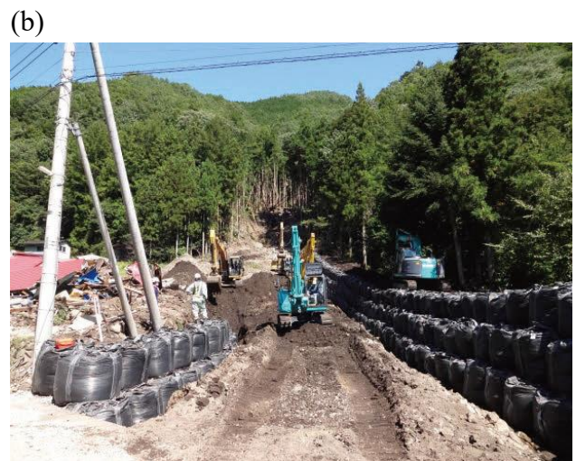
Fig. 15 Emergency construction (a) Right after the disaster (b) A temporary diversion channel is constructed with large sandbags
