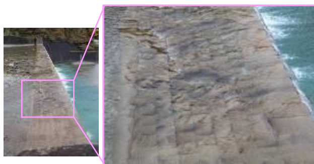
Fig. 8 Deterioration at the crest of the dam
