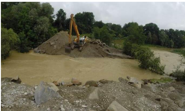
Fig. 2 Artificial levee breach (Source: VERBUND Innkraftwerke GmbH)
