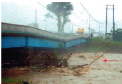
Photo 1. Accumulation of woody debris at a bridge pier.
