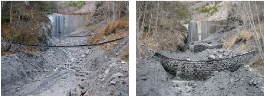
Fig 4: Multilevel Barrier Merdenson, Switzerland: 3 barriers in series empty (left) and filled (right).
