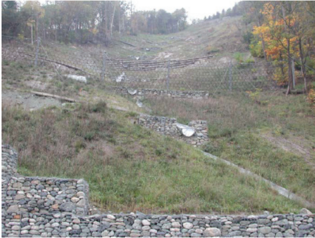
Fig. 6 : Detail view of a flexible catch fence
