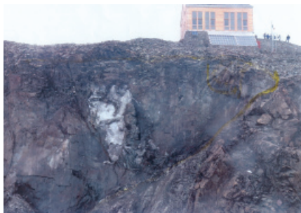
Fig.7: Massive ice outcroppig in the Marco and Rosa Hut rock fall scar (August 2003). Photo courtesy of CAI Valtellinese.
