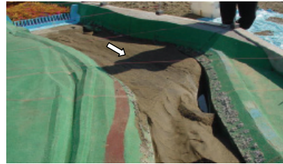
Photo 5. Scouring at an embankment leg downstream of a ground sill.
