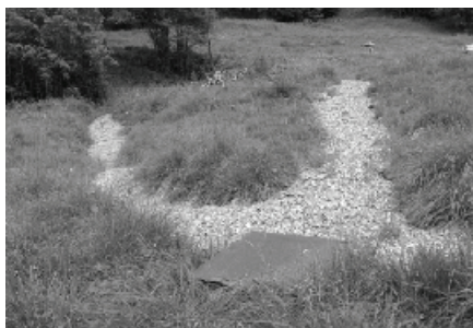
Abb. 8: Drainage zur Entwässerung instabiler Schichten. Fig. 8: Drainage system to stabilise the sliding layers of the slope.
