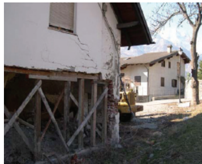
Fig. 4 : Oct. 2000 – Nus, house hit by the debris
